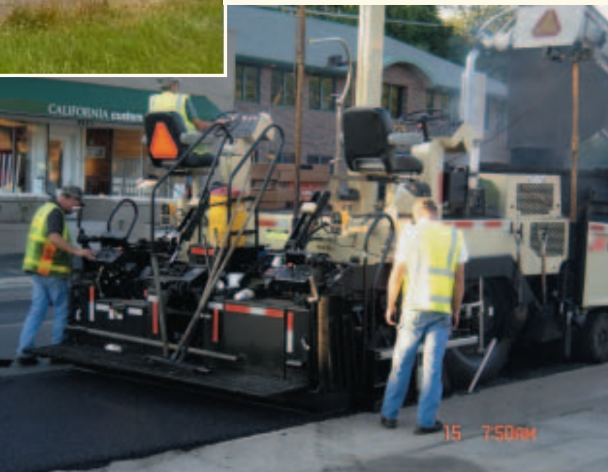
ace Construction Co. paves Route 100 in St. Louis during a nighttime job.
